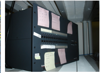
Figure 2. Video switch in the control room
